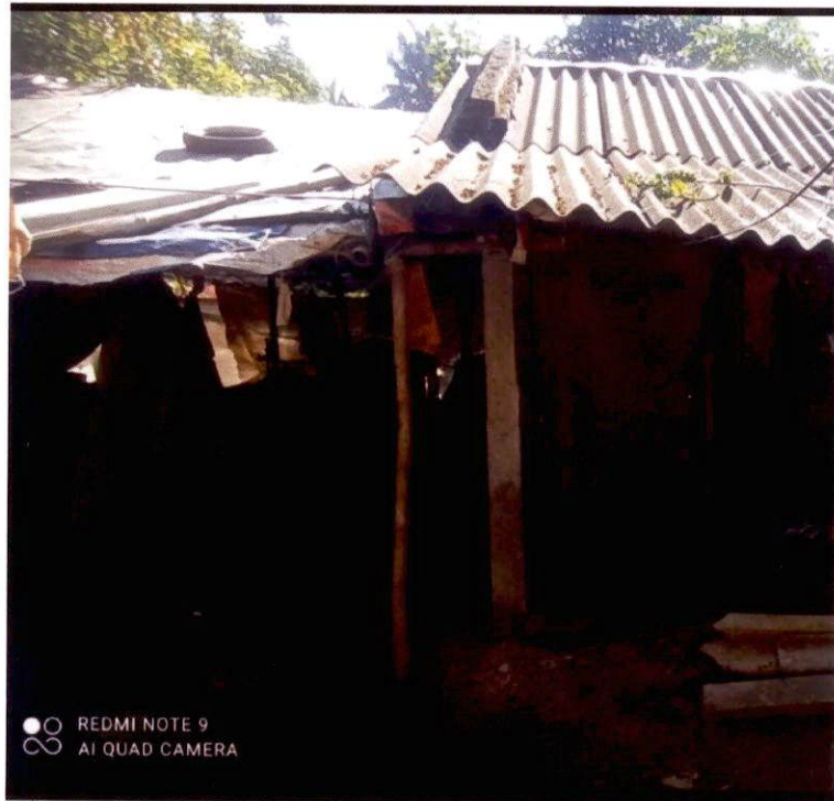
7. DILAPIDATED HOUSE OF SAPNA PATRA
